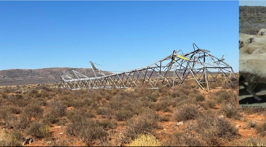
2024: Eskom pylons after windstorm – no electricity across large part of the Karoo for 15 days.
